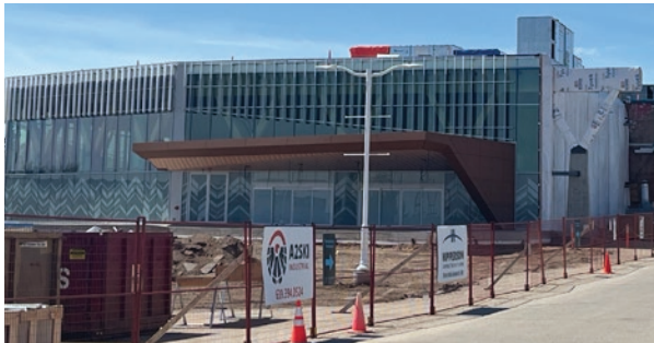
SIGA's renovation and expansion of its North Lights Casino in Prince Albert is well underway.
